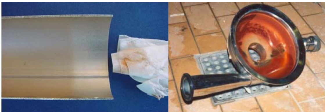
Figure 5.E-6 Rouging in a pure steam generator (source: Ciba Spezialitätenchemie AG)
